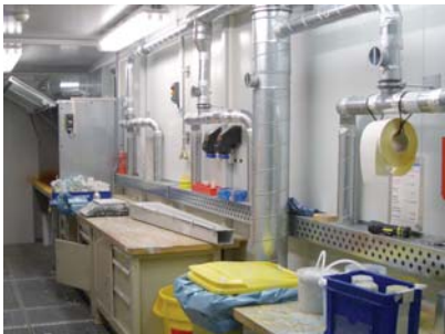
Interior view of the walk-in F90 Fire protection container with hazardous materials work station (in the background) and exhaust-ventilated workbench with ductwork.
