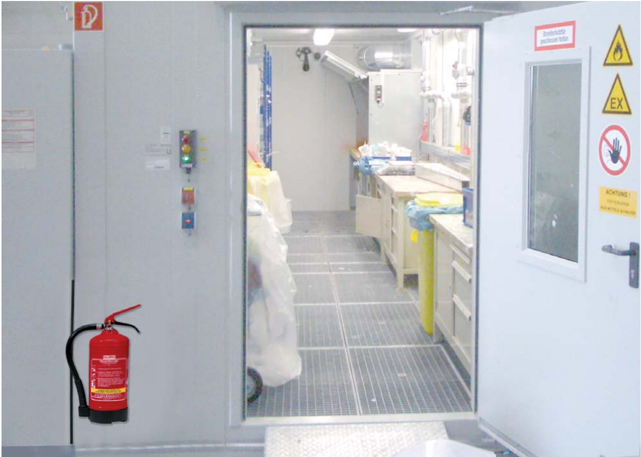
The walk-in F90 system with integrated hazardous materials work station and exhaust system in use. The storage unit has a T90 door with integrated F90 glazing as well as an alarm and signal lights plus a switch for illumination and a door restraint system.
